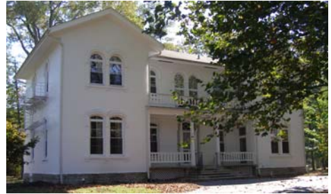
St. Angela Hall is undergoing renovation and will soon become the college's new administration building.
